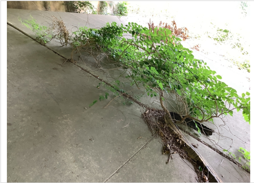
Vegetation growth between cracks in slope paving
