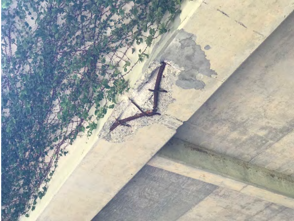
Closeup of damage under bridge
